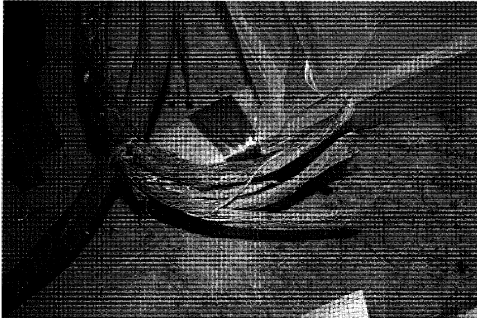
FIGURE 43. A photograph of the subject Distribution Cable from the subject Meter/Breaker Panel. (Image No.: NEC_1688)
