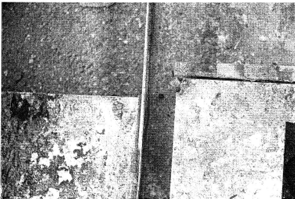
FIGURE 21. A photograph of the electrical fault activity present at the upper left corner for the subject Deadfront Cover for the Breaker Compartment positioned near the subject Barrier of the subject Meter/Breaker Panel. (Image No.: NEC_1414)
