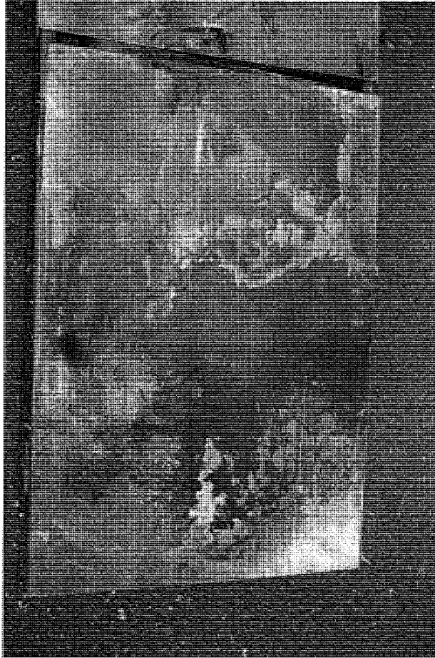
FIGURE 15. A photograph of the Breaker Compartment for the subject Meter/Breaker Panel. (Image No.: NEC_1202)
