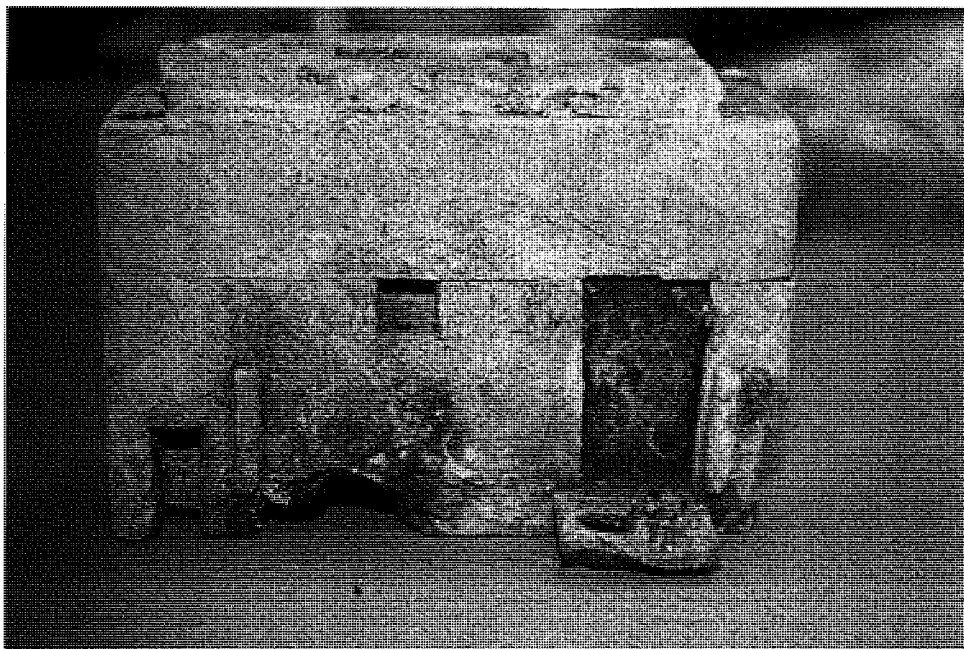
FIGURE 28. A photograph of the Load Side of the subject Circuit Breaker from the subject Meter/Breaker Panel. (Image No.: NEC_3699)
