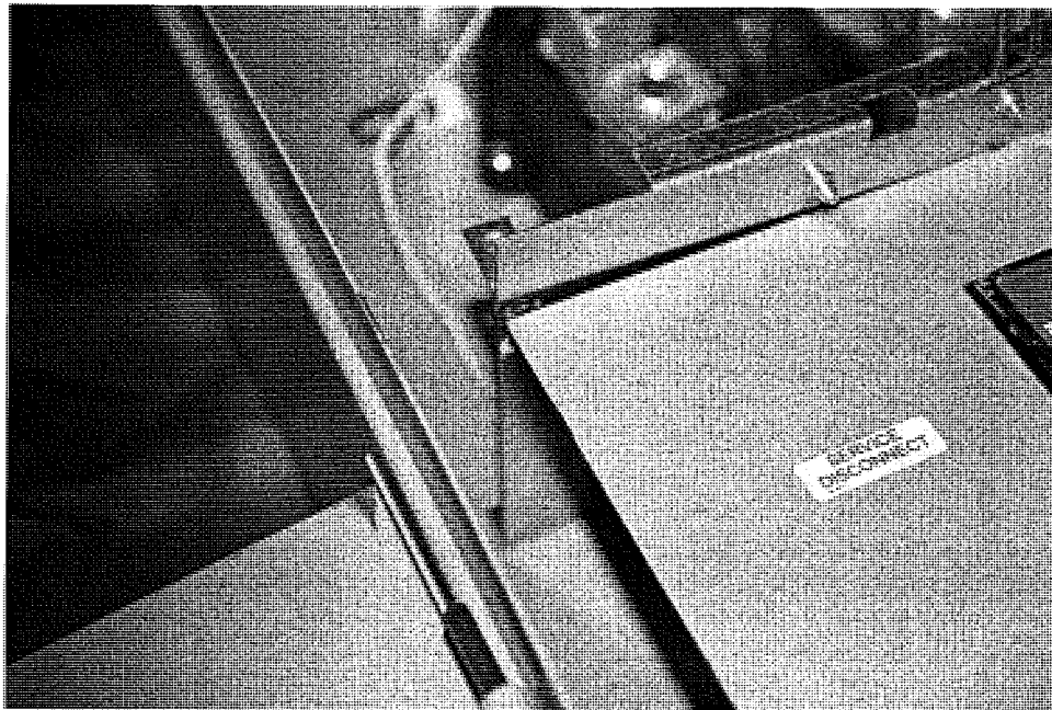
FIGURE 58. Photograph of the interior view of the Breaker Compartment for the exemplar Meter/Breaker Panel with the exemplar Wiring Gutter Enclosure removed and showing the edges of the exemplar Barrier and the exemplar Deadfront Cover. (Image No.: NEC_1727)
