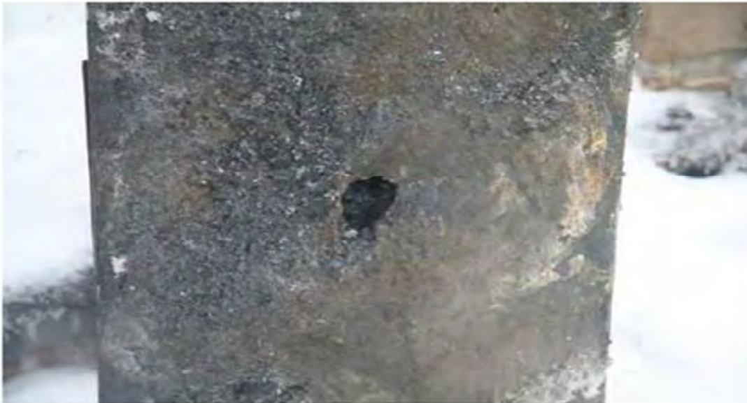
27. Hole in exterior rear side of enclosure
