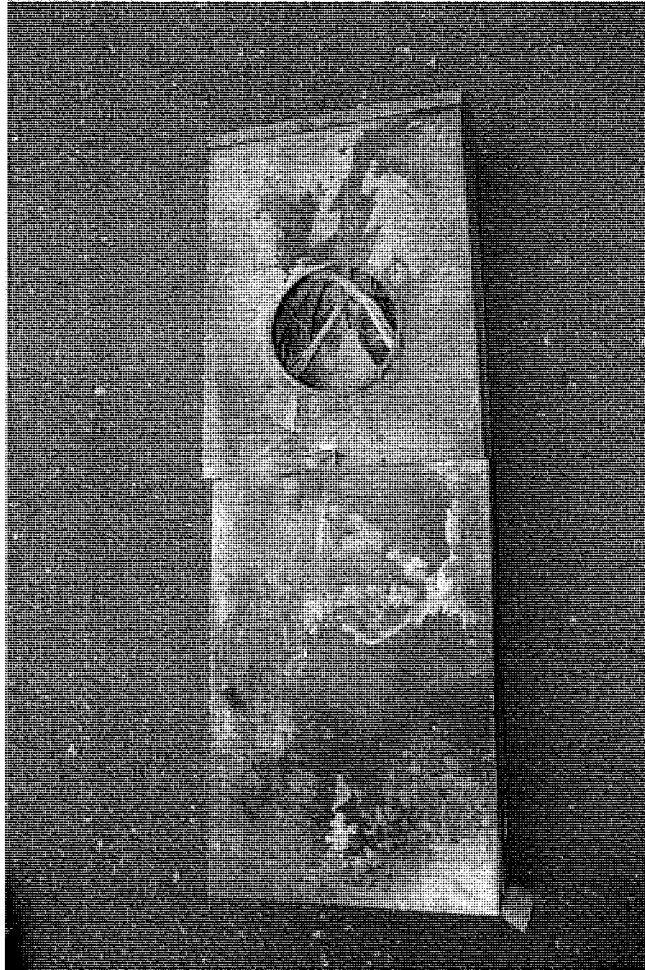
FIGURE 1. A photograph of the subject Meter/Breaker Panel. (Image No.: NEC_1184)
