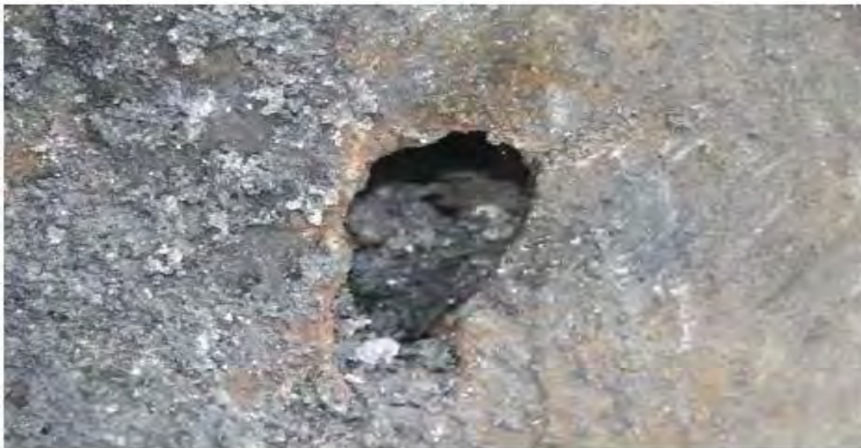
28. Closer view of hole in rear of enclosure
